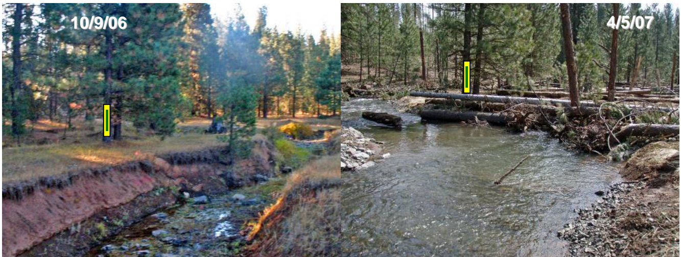
Figure 8. Ninety-five feet of new channel were constructed (visible on left side of 4/5/07 photo) and the stream was re-aligned into an old channel (Station 20+10).
