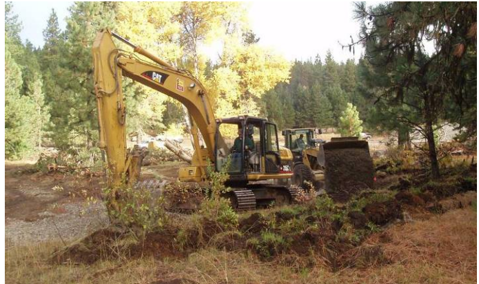
Figure 9. Salvage of sod mats and shrubs (foreground) and gravel fill for riffles (background)
