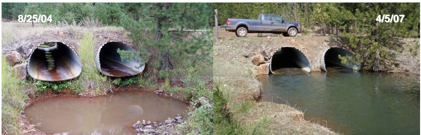
Figure 15. IXL Road crossing culvert outlets were backwatered by elevating the bed within the project reach.
