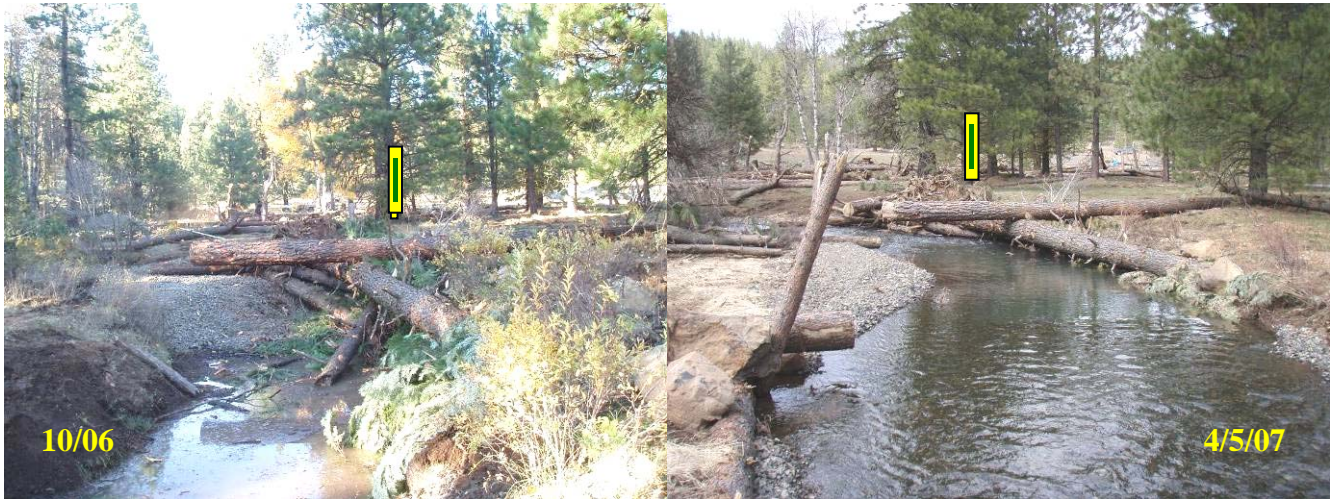
Figure 7. LWD jam constructed to enhance pool habitat complexity and reduce erosion (Station 13+40).
