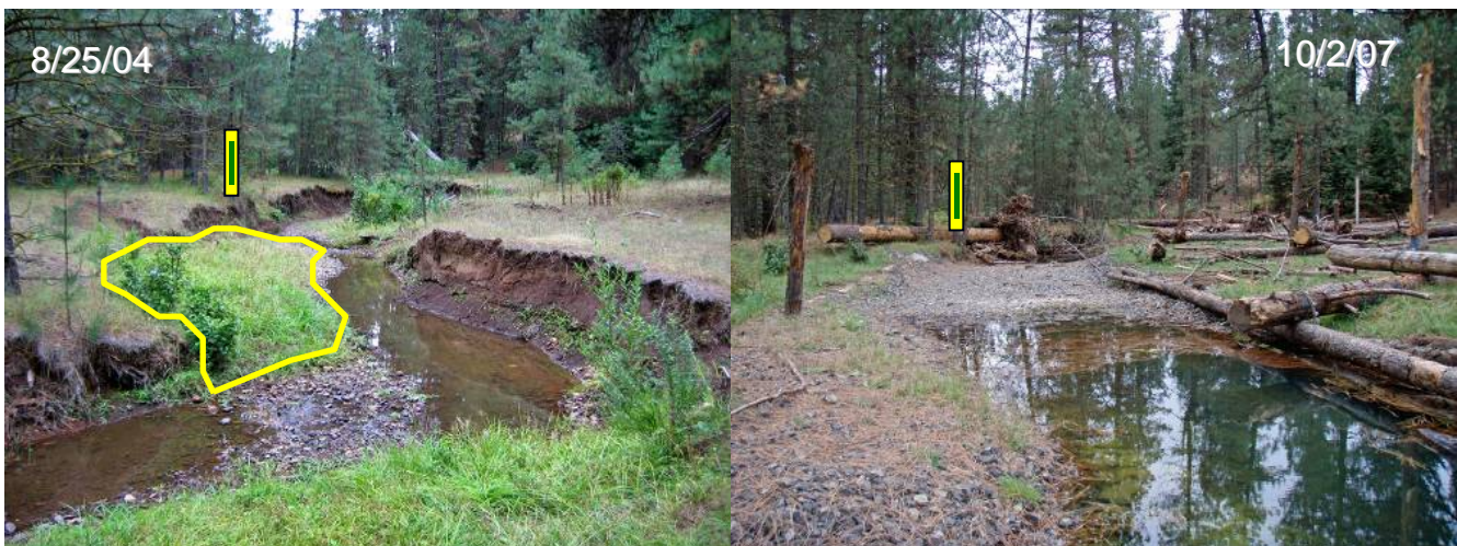
Figure 1. Pre- and post-construction photos of an isolated area (Station 10+80) within the project that showed signs of recovery prior to construction and were used to guide development of design dimensions.
