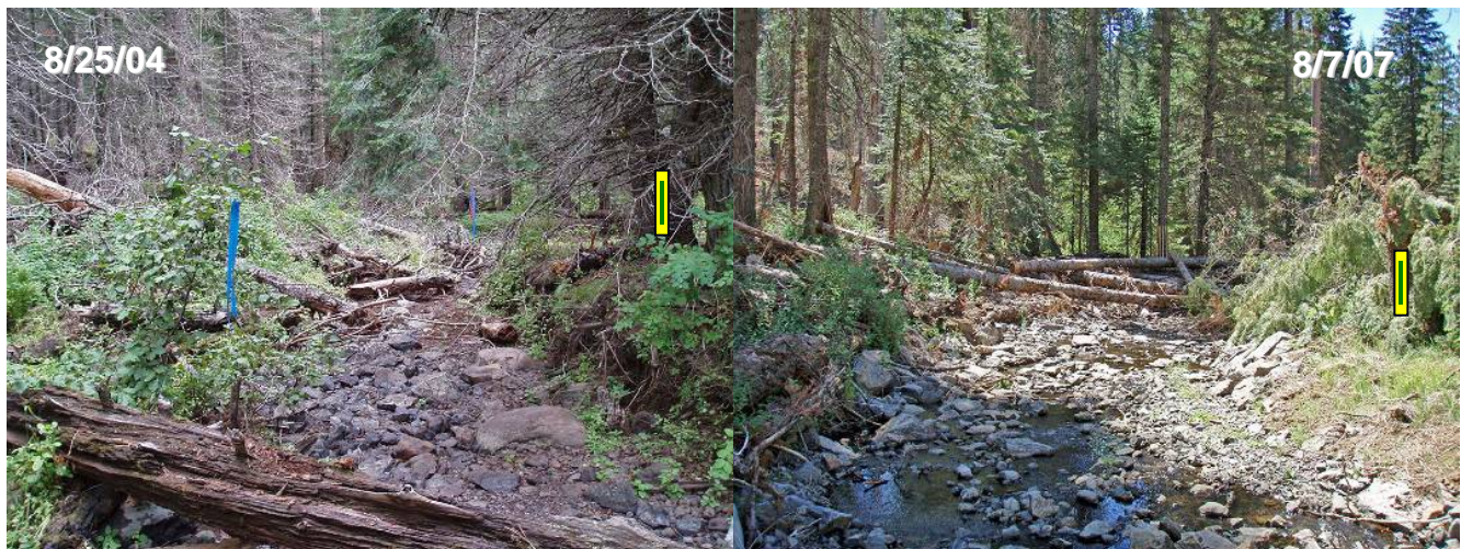
Figure 5. Upstream end of grade control riffle (Station 2+20) before (left) and after (right) construction.
