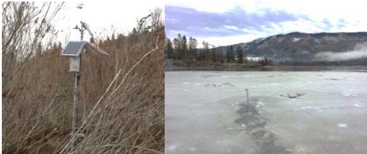
Figure 21. Mast and three-solar-panel array at East Delta (left) and February icing conditions.
