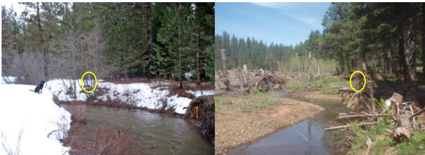
Figure 8. Tepee Creek Meadows Restoration – Phase 2 pre (left) and post riffle construction (right) and LWD placement, well (yellow circle) placement is consistent in both pictures although “post” picture is taken with a wider angle.
