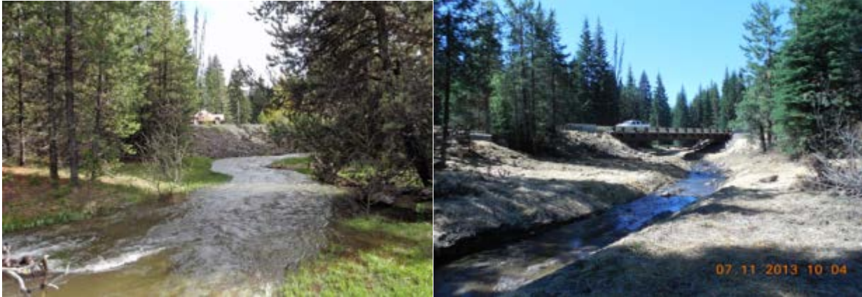
Figure 3. Upper Klickitat River In-channel and Floodplain Enhancement – Phase 3 pre (left) and post bridge installation (right) looking in the downstream direction above the 255 rd-xing.
