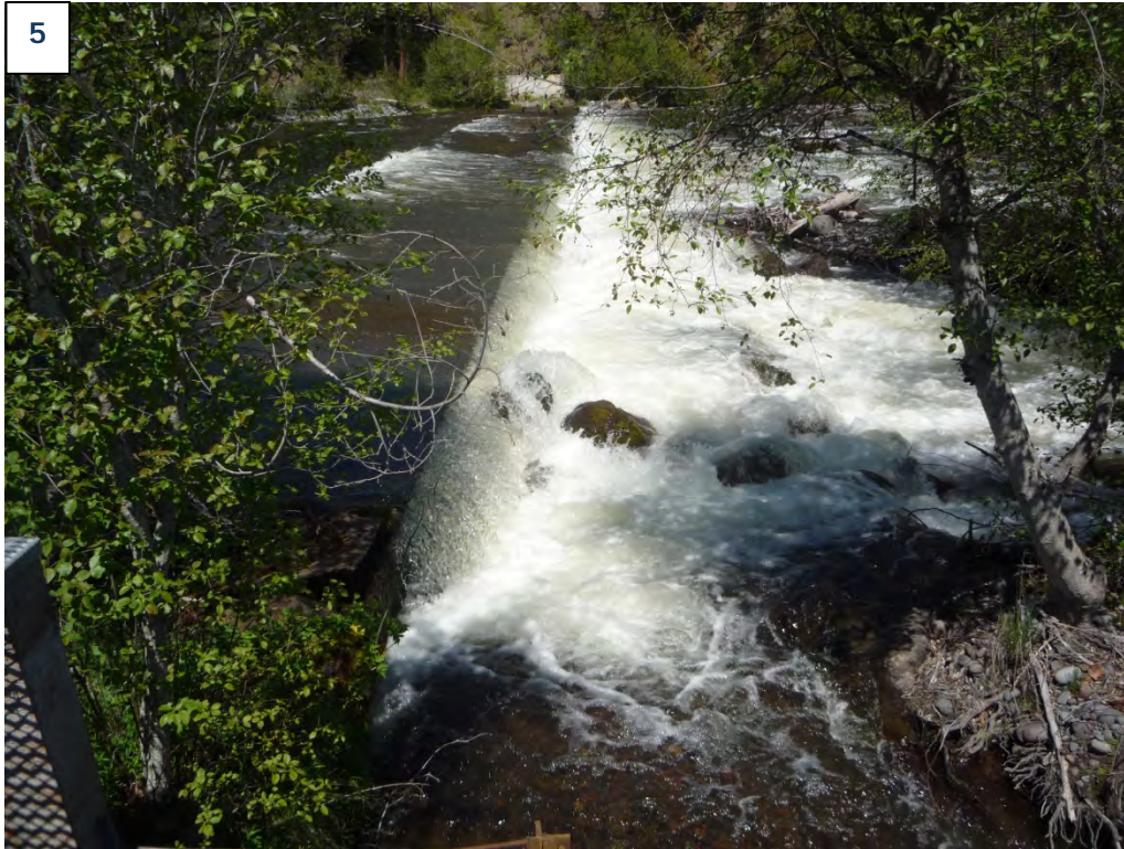
Klickitat River Concrete Sill
