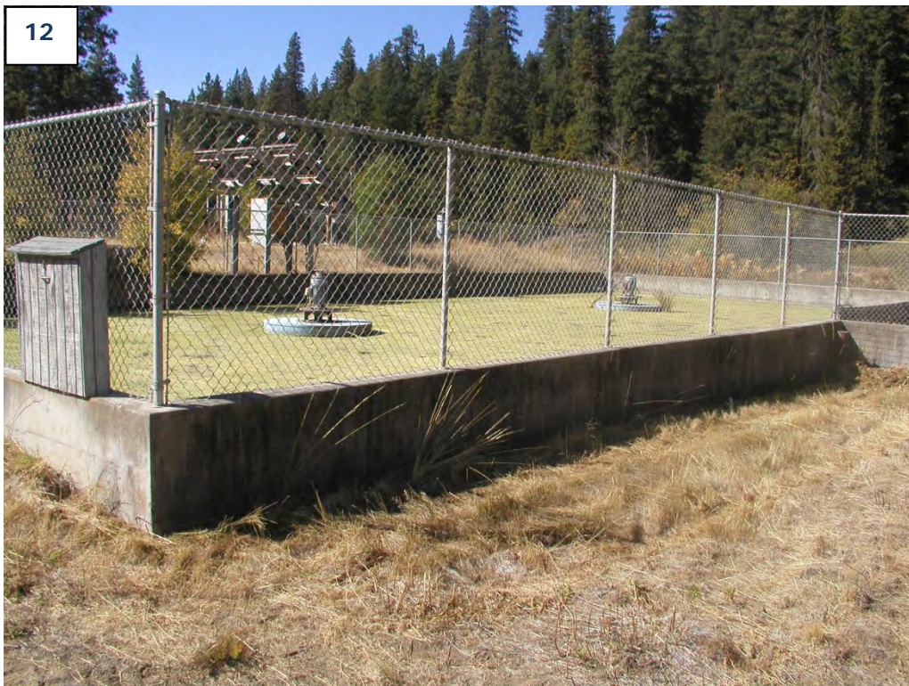
Pollution Abatement Basin
