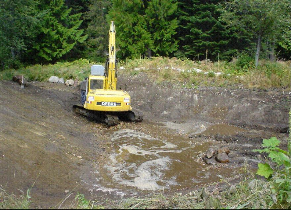
Figure F-2. Constructed Pond in Stream Channel - Mahar Acclimation Pond near Nason Creek, Wenatchee Basin
