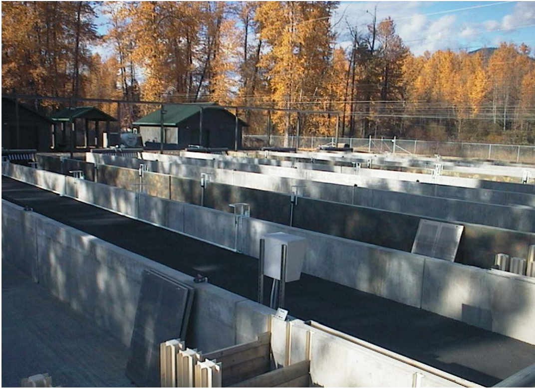
Figure F-4. Constructed Concrete Raceways - Easton Spring Chinook Acclimation Pond, YKFP
