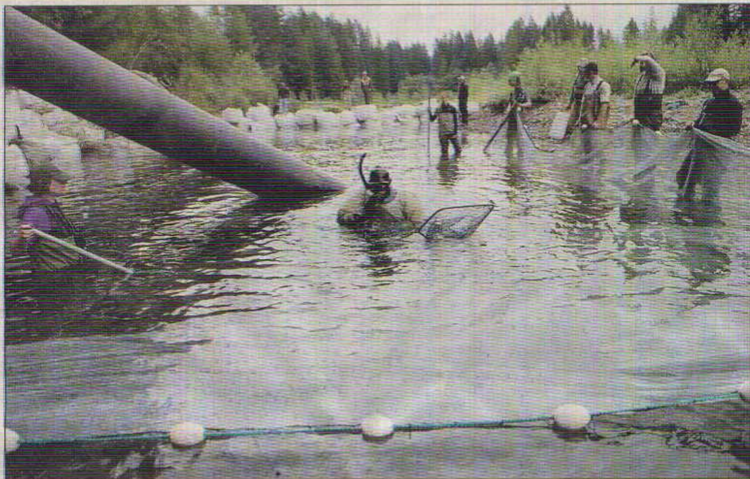
Snorkeler Kyle Marten and others try to net an elusive adult steelhead Monday in Trout Creek above Hemlock Dam. Fish above the dam were being moved downstream in preparation for piping the stream around the dam until it's demolished. The 20-inch fish got away. Photos by STEVEN LANE/The Columbian
