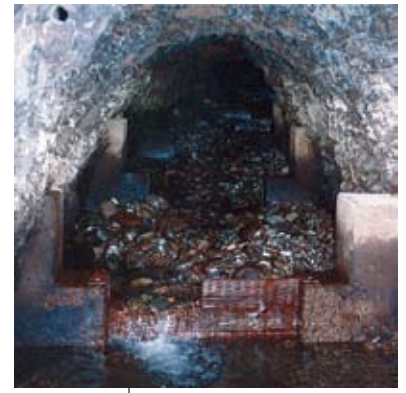
Prior to the retrofit, the salmon tunnel was filled with cobble and didn't pass deep enough water for salmon to navigate its depth.
